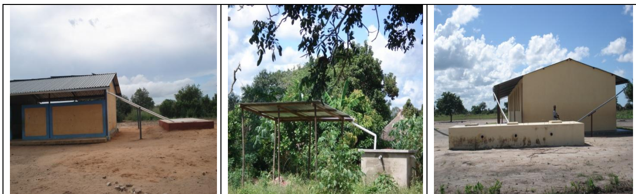
Figure 16: Example of tanks connected to the roofs of houses in Nova Mambone.
